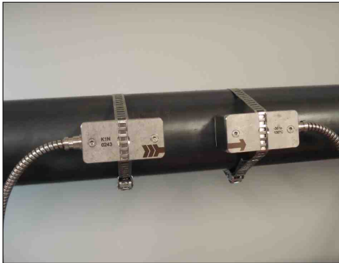
Transducers mounted using strap and clamps
